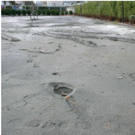
Liquefaction at Central business district of Christchurch Earthquake, New Zealand
